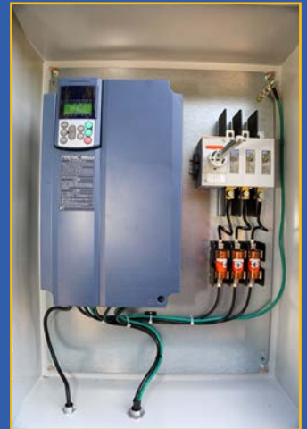
Interior view of electrical enclosure - viewing safety disconnect switch, fuses and Fuji Frenica Mega Programmable Variable Frequency Drive that has all the ground fault and short circuit protection, the VFD shown will prevent electrical usage spikes which should help reduce electric energy costs.
